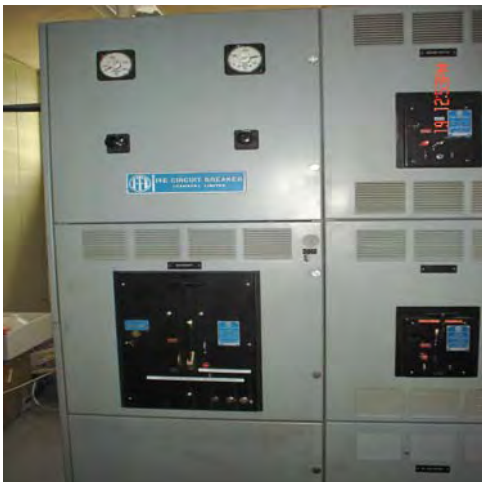
Original controls for building power, replacement parts difficult if not impossible to find
