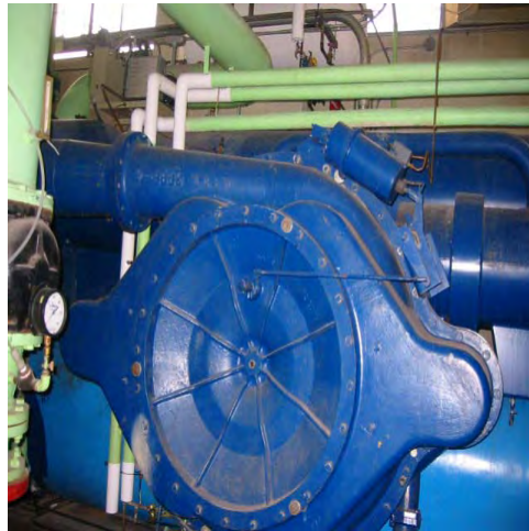
R11 Chiller – end of life
