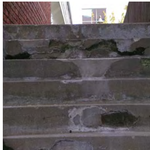
Spalling on stairs
