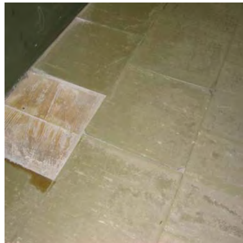
Missing vinyl floor tiles
