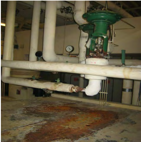
Asbestos insulated pipes
