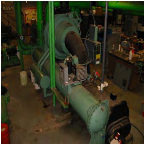
Original 1969 boiler – contains R11 refrigerant – beyond life expectancy
