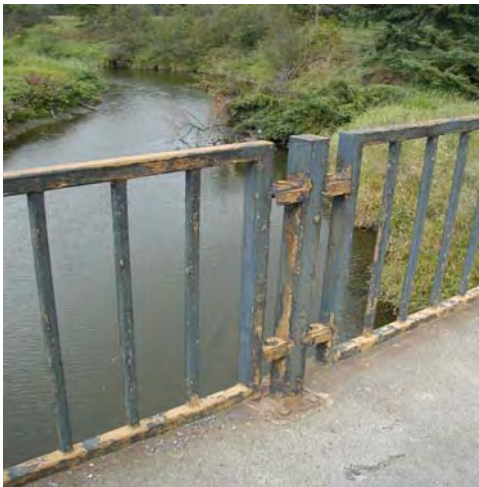
Bridge railing and concrete deterioration
