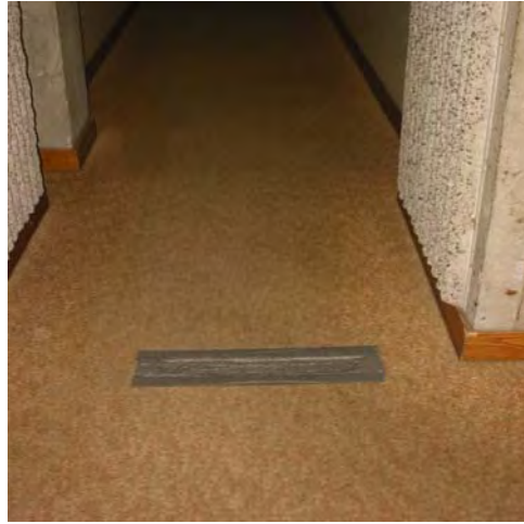
Torn corridor carpet repaired with duct tape
