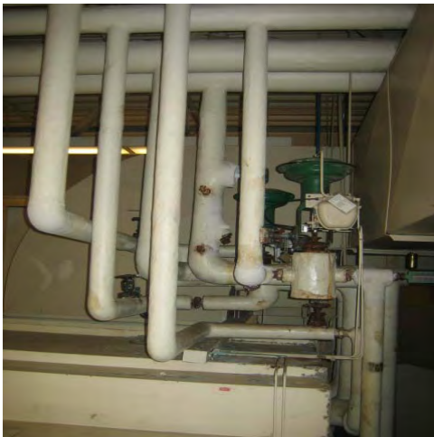
Asbestos insulated pipes
