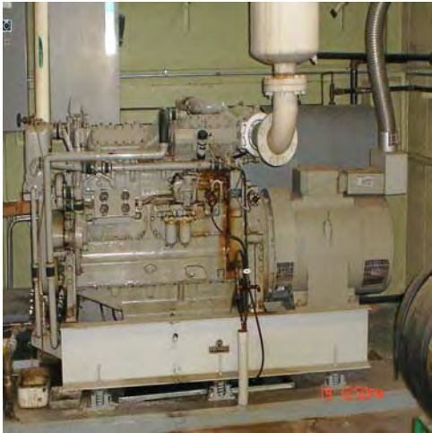
Antiquated diesel generator for emergency lighting
