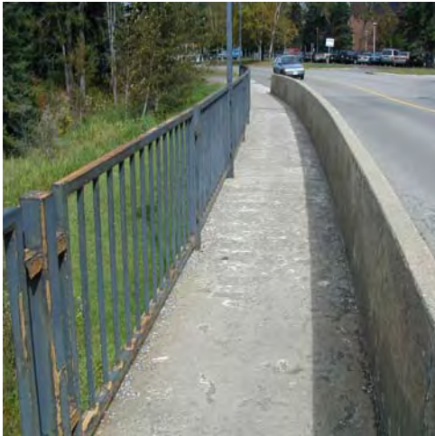
Bridge railing and concrete deterioration
