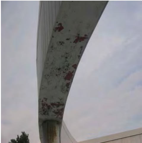
Moisture damaged soffit
