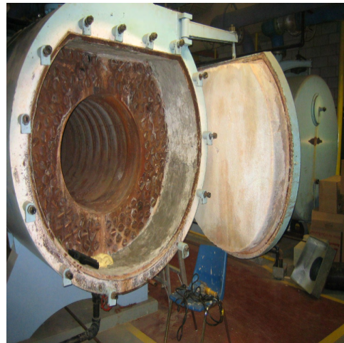
40 year old boiler – beyond useful life expectancy
