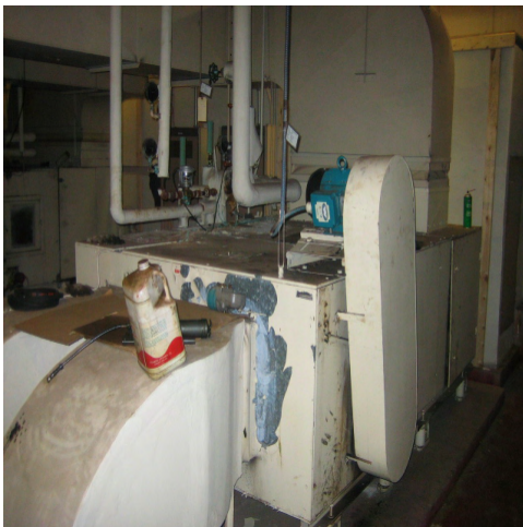
Original air handling units – beyond useful life expectancy, poor efficiency
