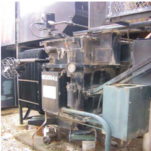
Original 40 year old transformer – beyond life cycle
