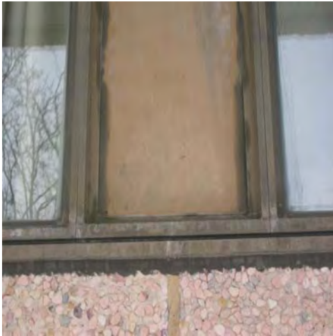
Damaged window seals
