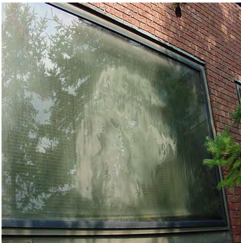
Damaged window seals
