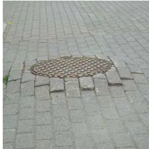
Settling of brick work
