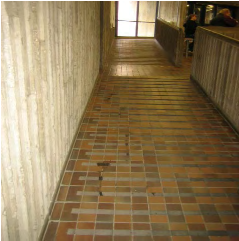
Repurposed service ramp – not to code
