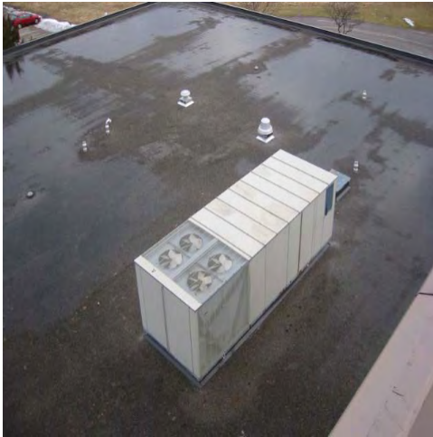
Rooftop HVAC unit – end of life
