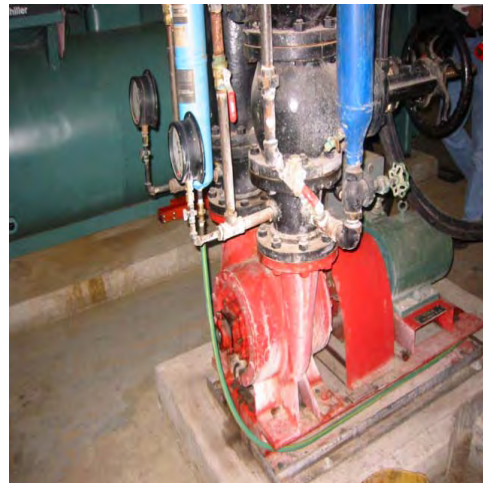
Heating system pumps – end of life
