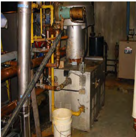
Antiquated original 1969 boiler
