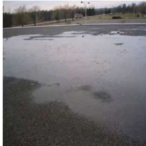
Improper roof drainage
