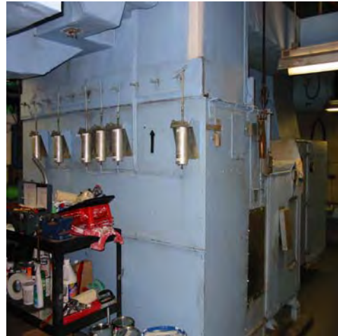
Original 1969 HVAC unit
