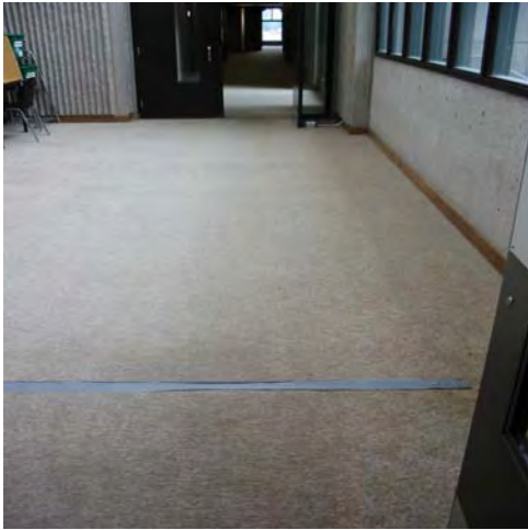
Damaged carpet seams in student study area
