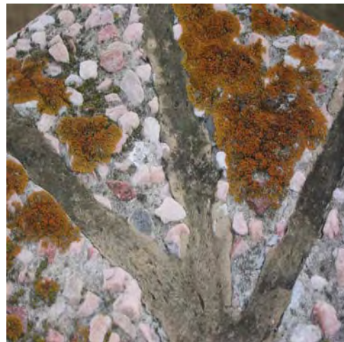
Damaged soft joint sealant on exterior walls
