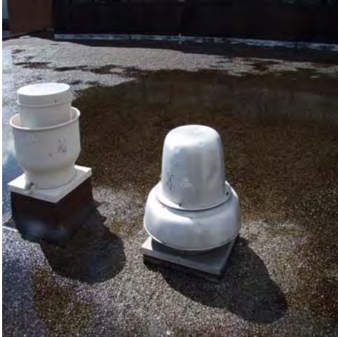
Ductwork and exhaust fan system part of Science and Technology lab - not to standards
