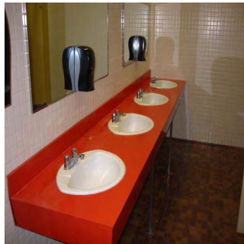
Old washrooms / poor water conservation
