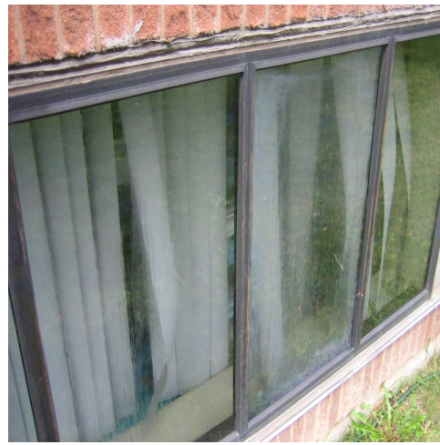
Broken window seals, compromised thermal efficiency, weather seal and viewing properties
