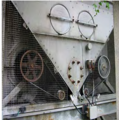
Antiquated cooling tower
