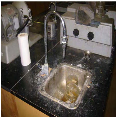
Electrical GFCI receptacle required
