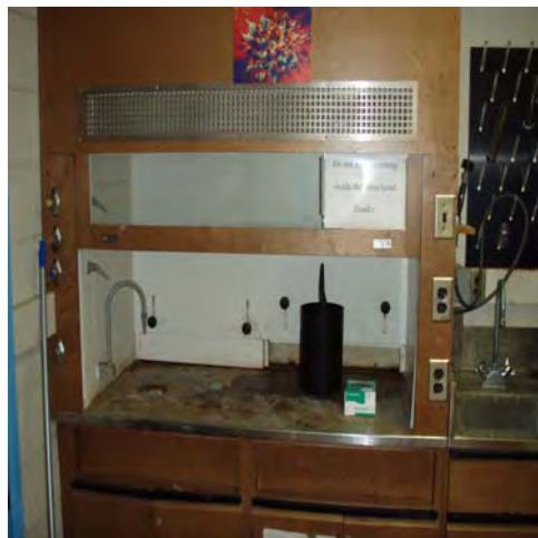
Science and Technology lab fume hood not to standards
