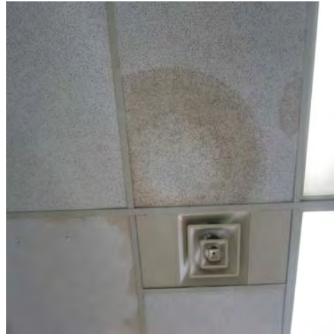
Water damage to ceiling tiles
