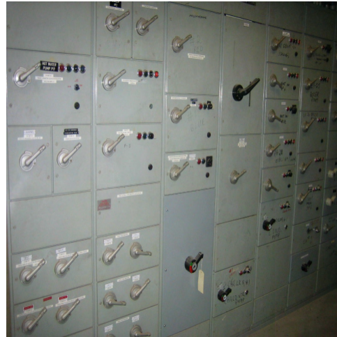
40 year old electrical switch panels – subject to catastrophic failure due to age
