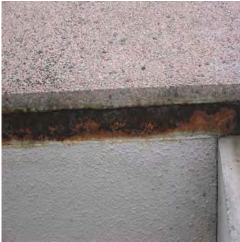
Rusted steel lintels on exterior walls
