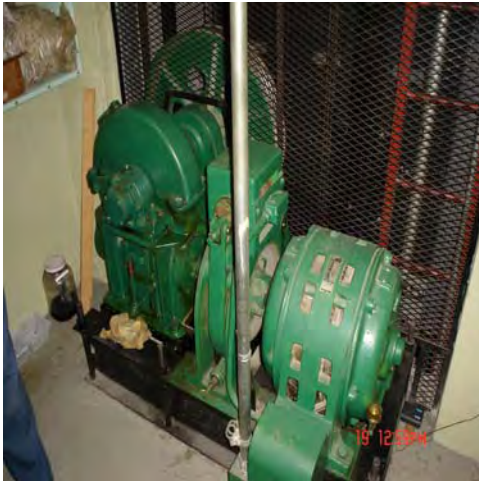
1967 elevator drive system
