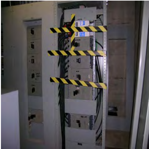
Antiquated electrical panels
